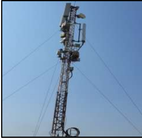
Plate 1: The communication tower (self-supporting tower)
